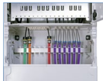
In all pillars, microducts are terminated with a gas block in the base.
