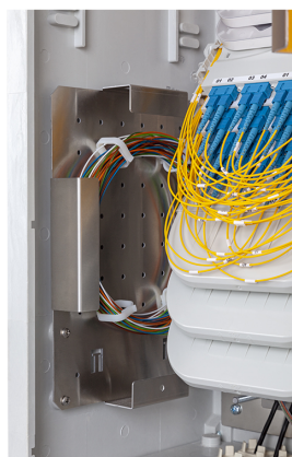
Fiber Distribution Hub MDP EL 144/288
