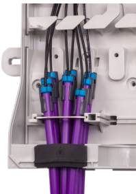
Microduct Termination in the Box
